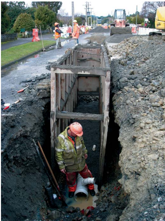
Construction of Cockburn Street sewer replacement. Though only laid as recently as 1954, the existing sewer experiences high levels of inflow and infiltration and causes problems on a regular basis.
