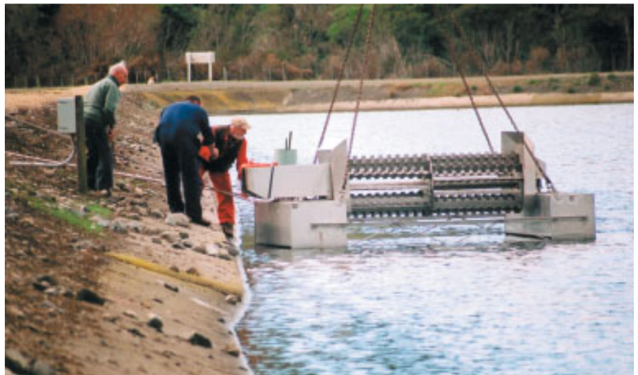
The first of the five new cage aerators installed in the oxidation ponds at Homebush is lowered into place. Two have been installed in each of the primary treatment ponds and one in the secondary treatment pond.
