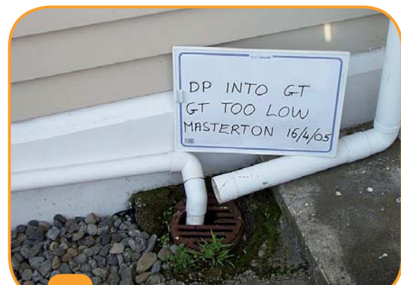
21 Typical gully trap faults which causes rainwater inflow to the sewers
